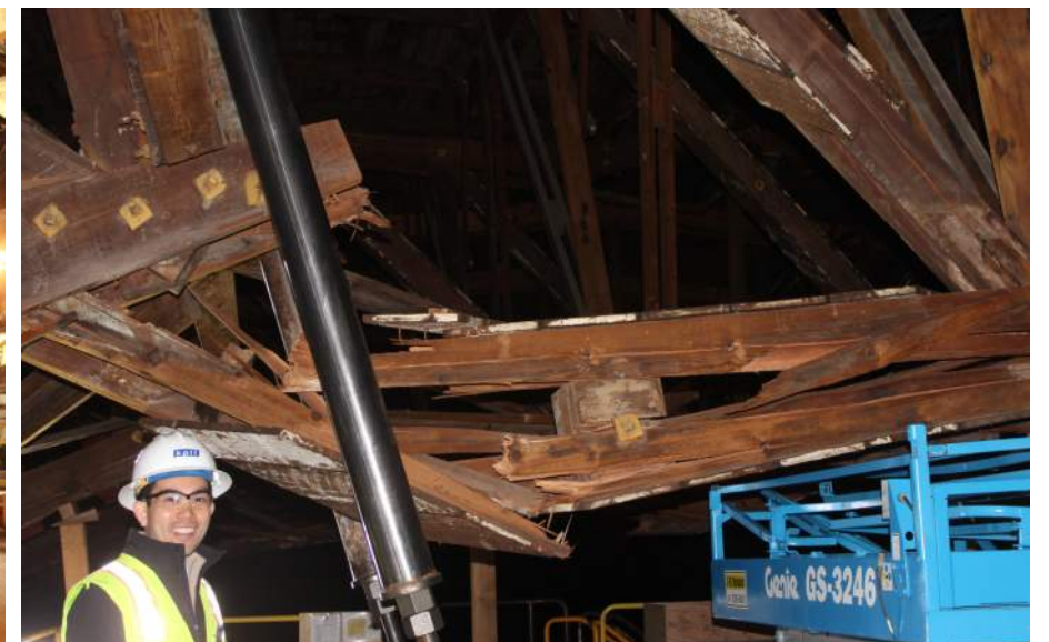
Damaged chord member viewed from access tower
